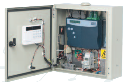
Squirrel 2020 in an electrical enclosure
